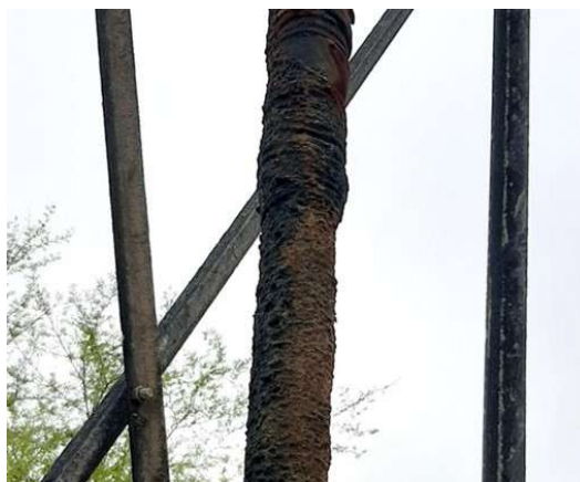
Figure 1. Metal pipe used in water extraction corroded by H_2S .
