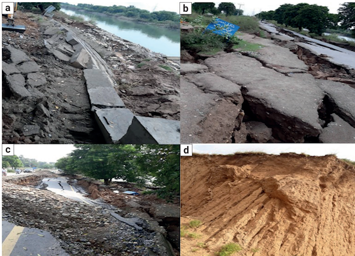
Figure 5. a, b, c showing liquefaction effect and subsidence in saturated clay along the UJC due to earthquake shaking at different locations, and d) an exposed clay deposit in the area.
