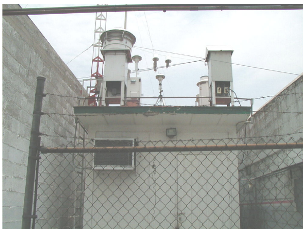
FIGURE 1. Typical facilities for environmental monitoring of metropolitan network where lichens were.
