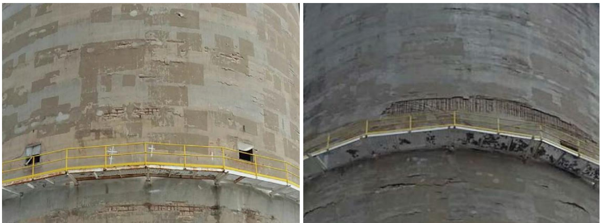
Figure 3. Exposed steel reinforcement, corrosion, concrete spalling and multiple rectangles indicating the sites of previous localized repairs.
