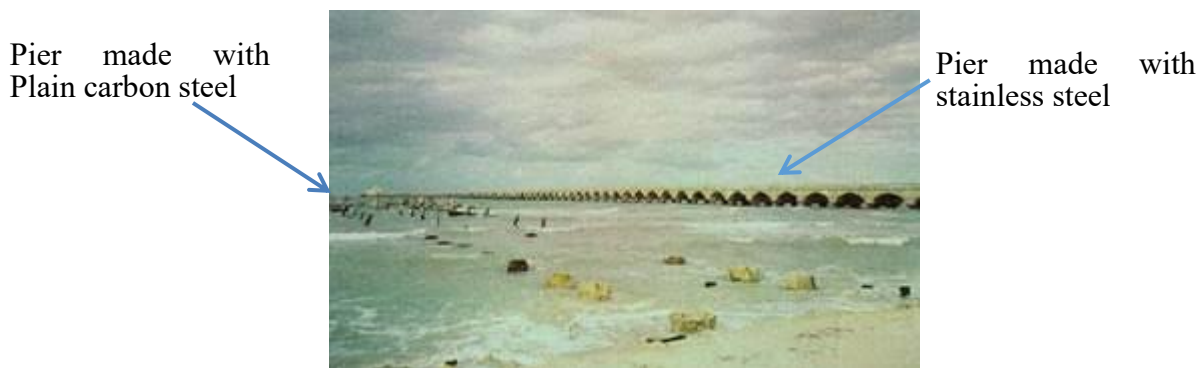
Figure1. Comparison between the pier with structures made with stainless steel (right) and the pier with structures made with carbon steel (left) (Klueh, R. L., & King, J. F. 1982).
