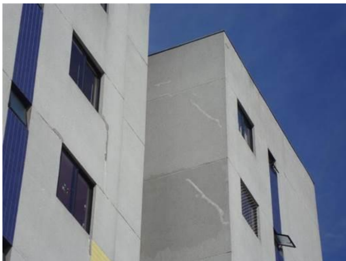
b) Structure movement fissures.
