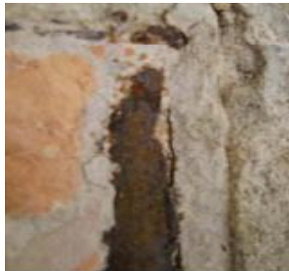
Figure 5. Columns' longitudinal reinforcement eroded (corrosion).
