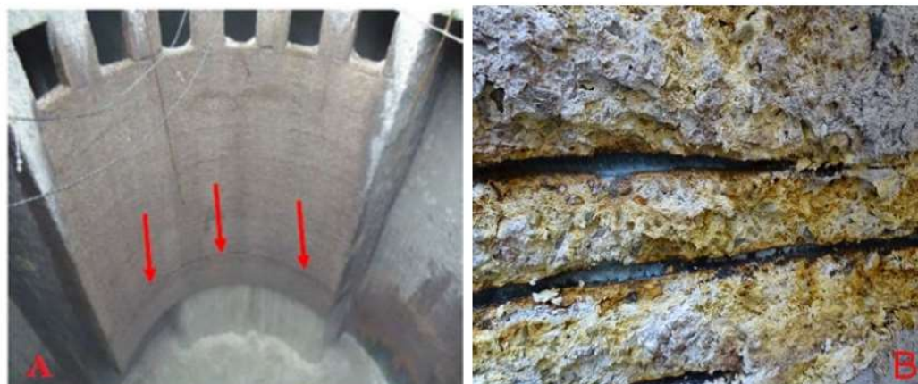
Figure 1. (a) wet-well (b) Degradation of concrete and steel bars observed by site inspection
