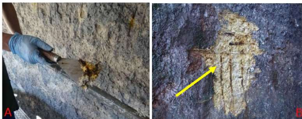
Figure 2. (a) removal of the degraded concrete layer using a spatula and (b) parts of completely reinforcement dissolution
