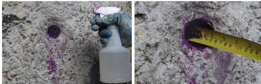
Figure 4: wet-well's wall - alkaline concrete
