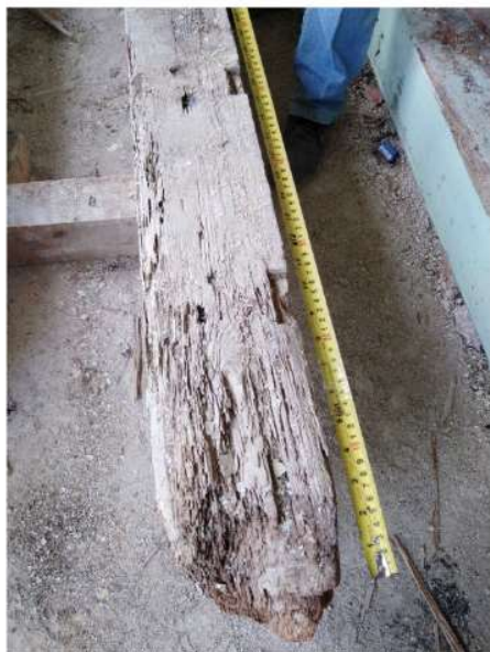
Figure 7. Measure of the affected beam section with Steel tape
