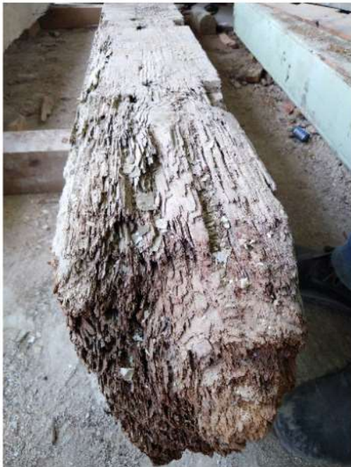
Figure 5. State of the beam heads
