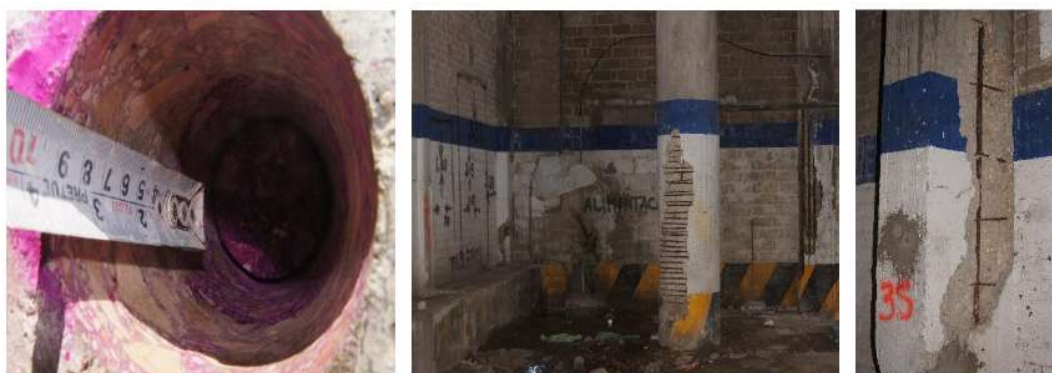
Figure. 3. Carbonation and detachment of concrete.
