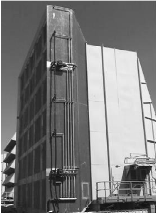
Figure 5. OMM cooler installed on gas turbine unit 3 of Kerman C.C.P.P, Iran.
